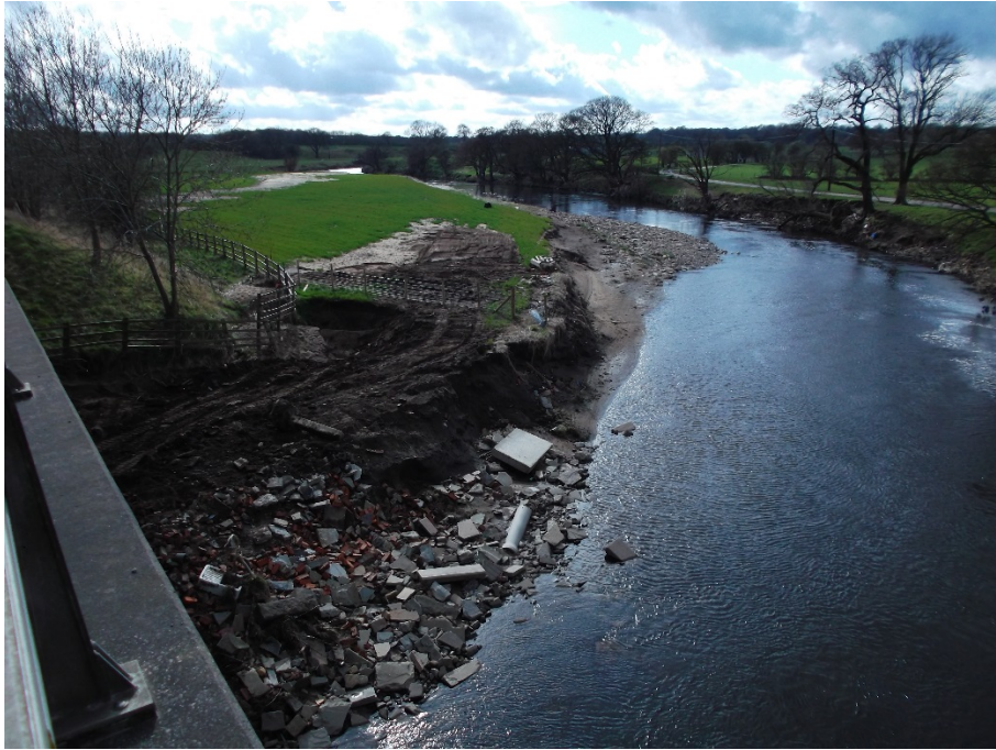
The Deep pool showing the scars of the flood in 2015
